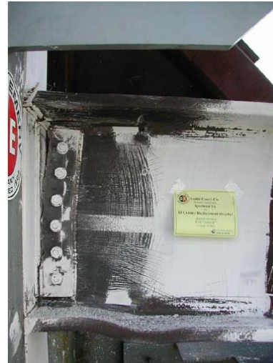
FIGURE 16. Ductile yielding and of beam (SSDA 2005)
