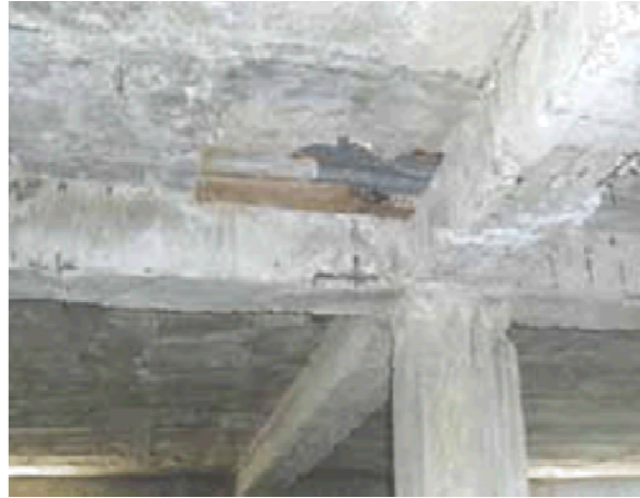
Figure 2 Example of poor construction in Haiti
