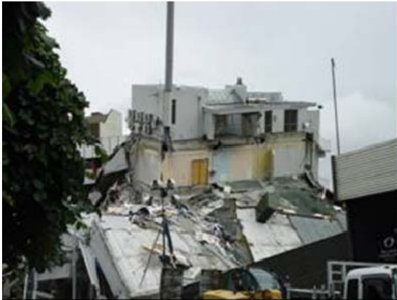
Figure 4. Collapsed nonductile concrete building in the CBD
