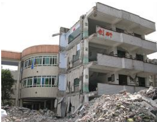
a. Collapsed building; note the standing stairway
