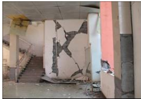
b. Cracked wall
