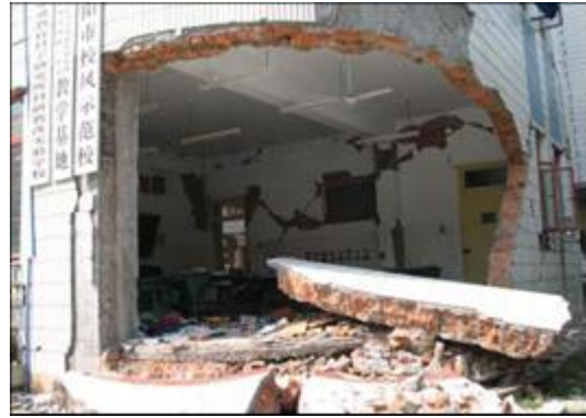
b. Collapsed first floor
