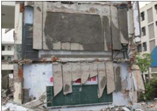
a. Collapsed floor planks
