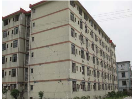
b. Cracked wall
