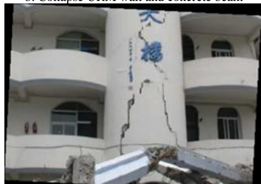
d. Cracked URM
