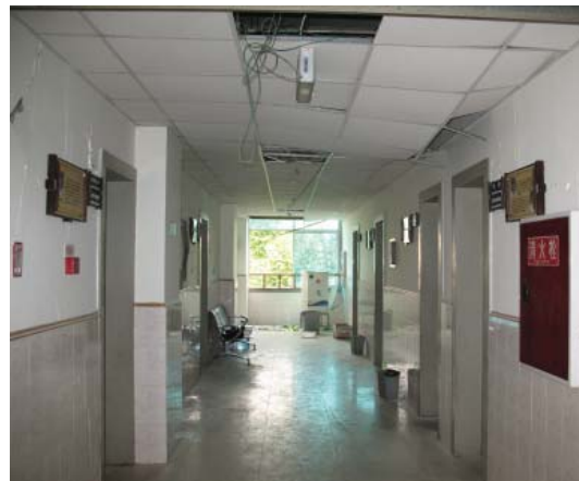
b. Nonstructural damage
