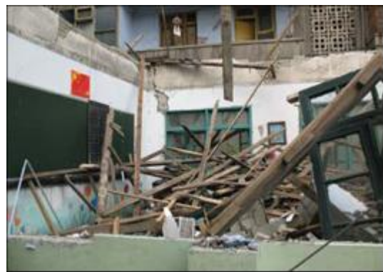
b. Collapsed first floor
