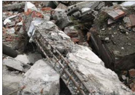
b. Collapse URM wall and concrete beam
