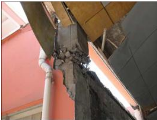
a. Column flexural failure
