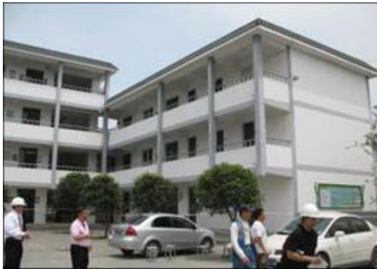
a. Minor pounding damage
